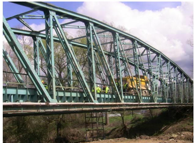
Fig. 4 View of the bridge during the phase of examination under test load
