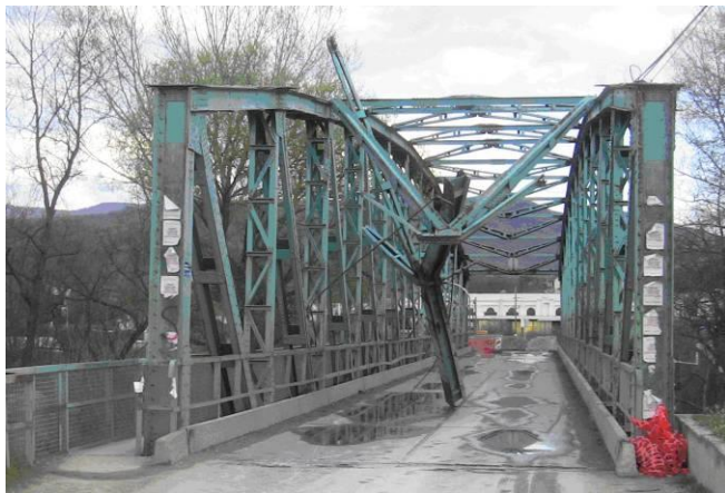
Fig. 2 Damages of the bridge
