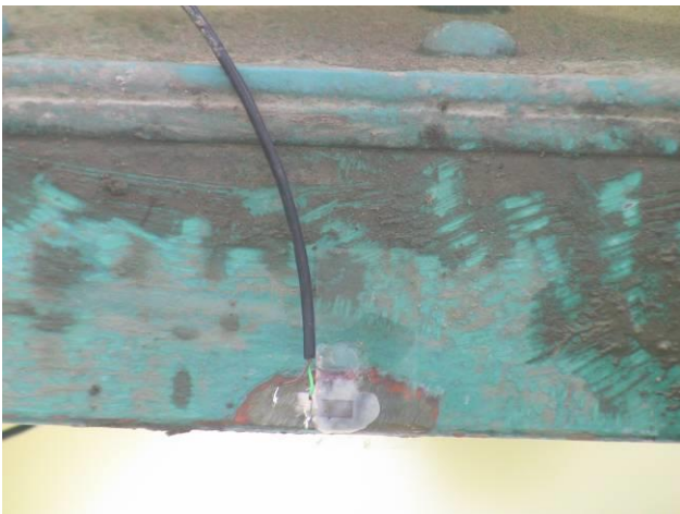
Fig. 7 Strain gauge M2 set on the bottom chord member in the midspan
